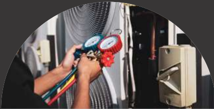
Air Conditioning Equipment
