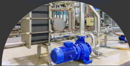
Heat Exchangers, Pumps & Equipment
