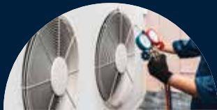
Innovation & Emerging Technologies in HVAC
