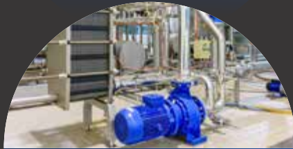
Heat Exchangers, Pumps & Equipment
